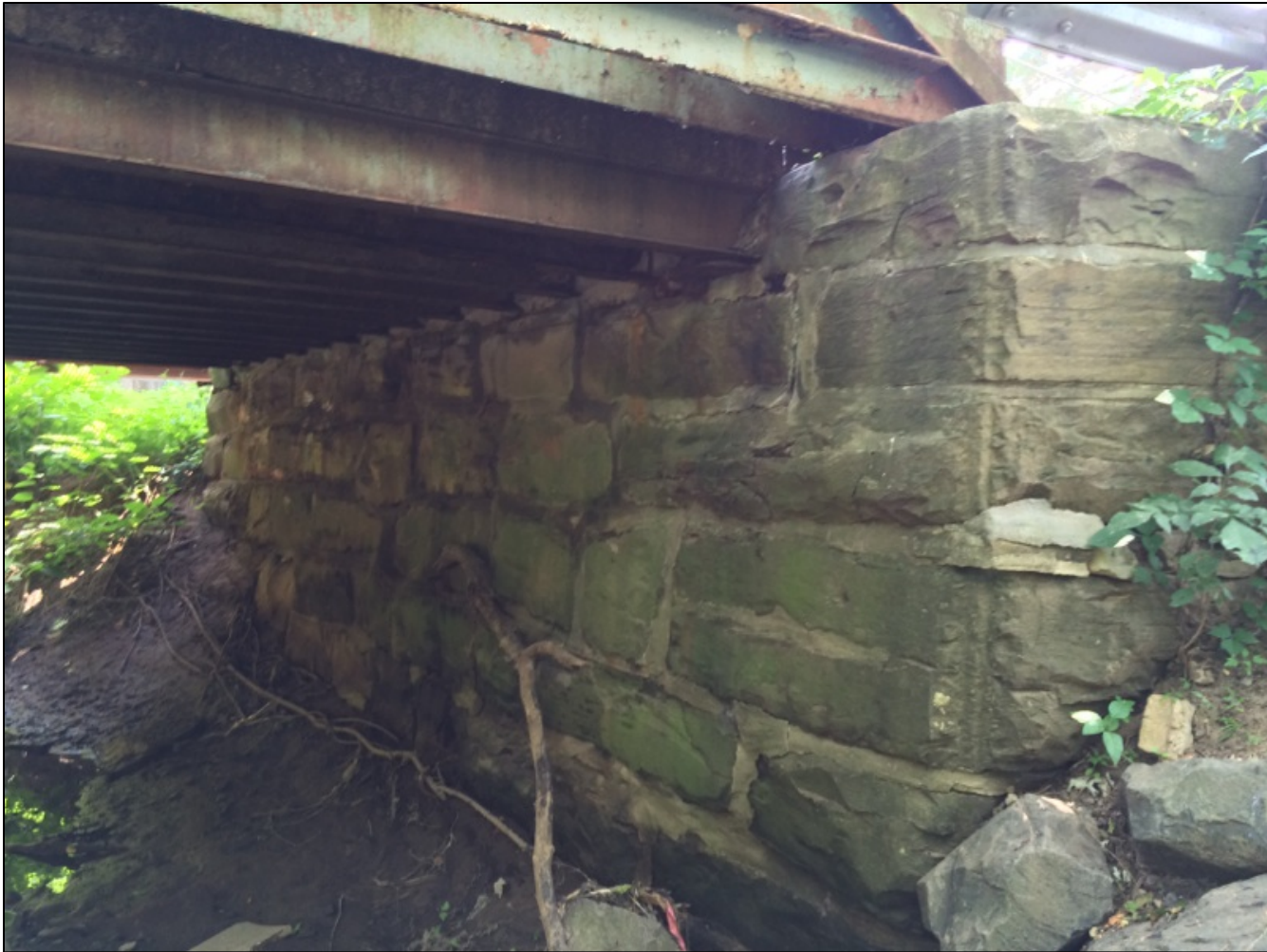
Enclosure 7. Jefferson Avenue Bridge looking to southern abutment. The bridge abutments will remain in place. Photographer: Lynn Rakos, July 2014.
