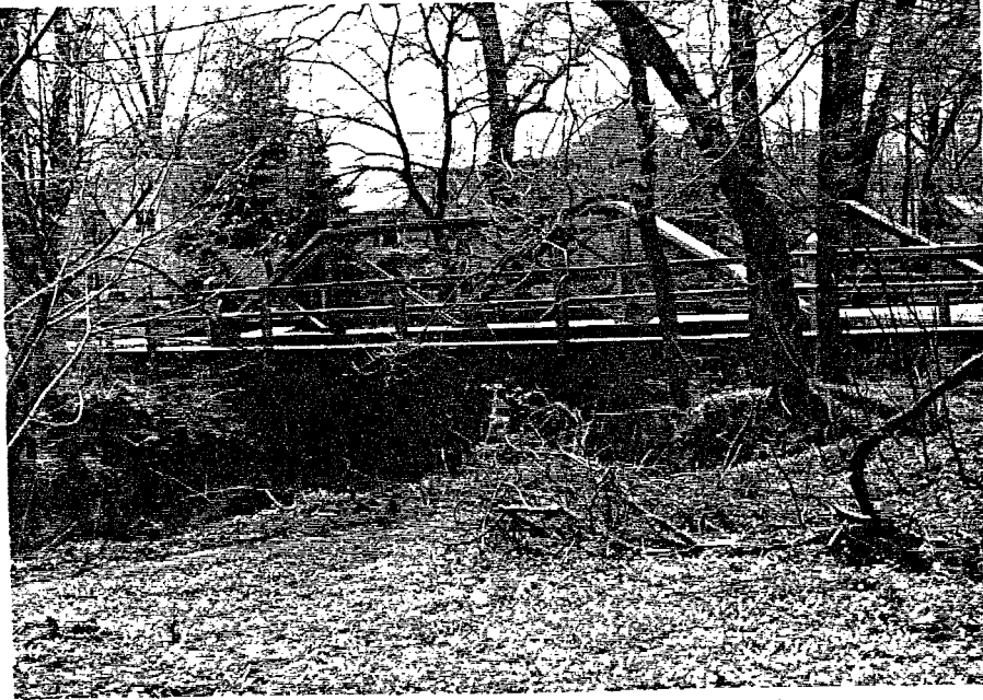
Plate 6.42 Site 49, Jefferson Avenue Bridge over Green Brook, City of Plainfield, Dumellen Borough and Green Brook Township; view looking southwest at the east elevation (Photographer: Lynn Rakos, April 1990).
