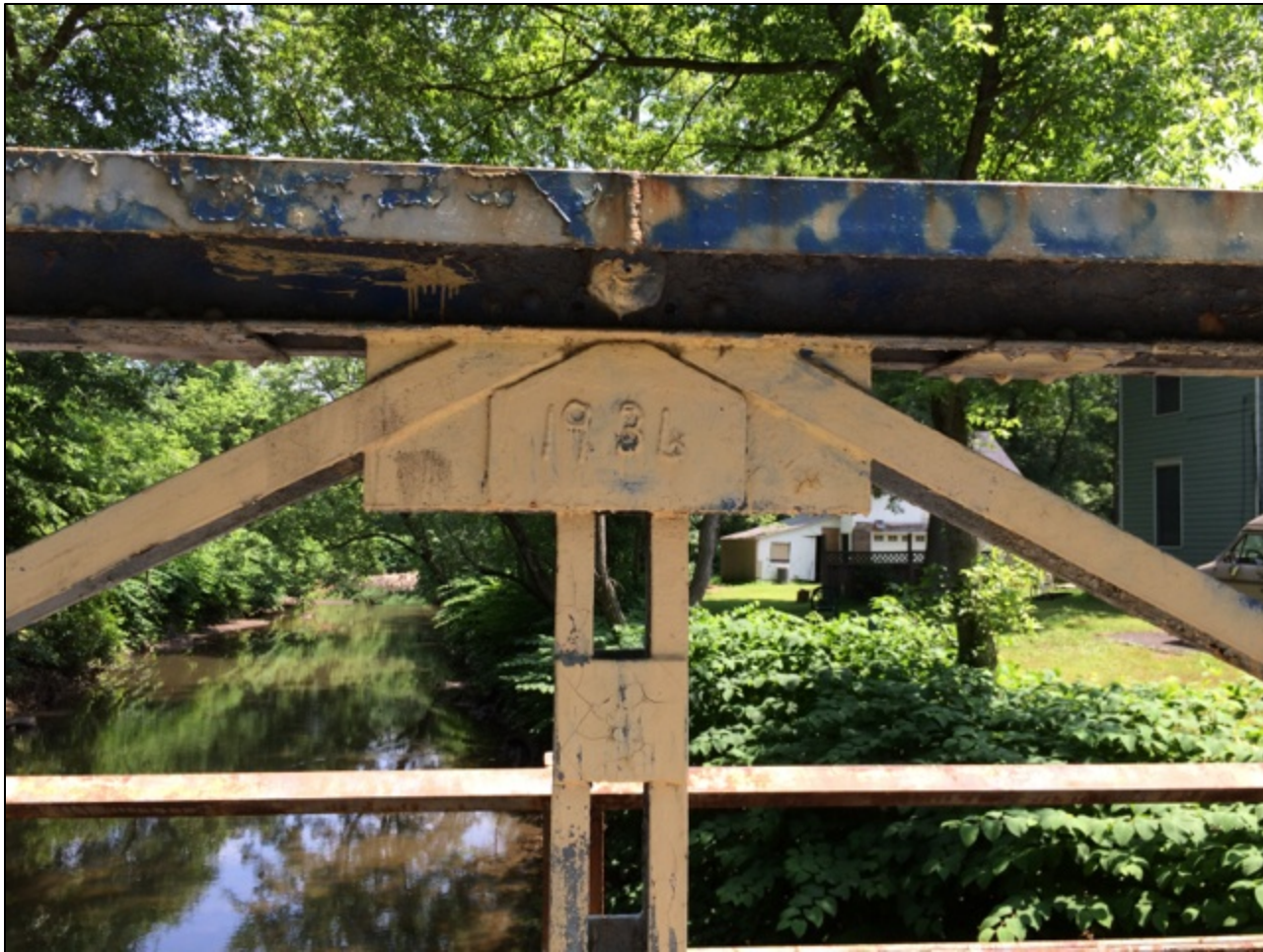
Enclosure 8. Jefferson Avenue Bridge view to east truss line of handmade plaque reading “1936;” likely a year the bridge was rebuilt or repaired. Photographer: Lynn Rakos, July 2014.
