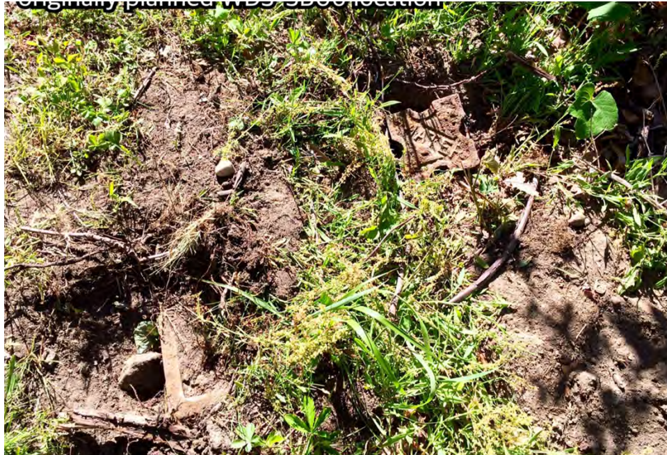
Waste Disposal System. Portion of water line found in vicinity of the original RI Work Plan WDS-SB06 location, June 2016.
