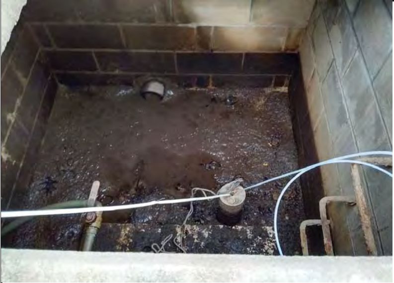
Photo 3. 3001-MW01: 4-inch casing with 1-inch PVC, 6-inch drain pipe.
