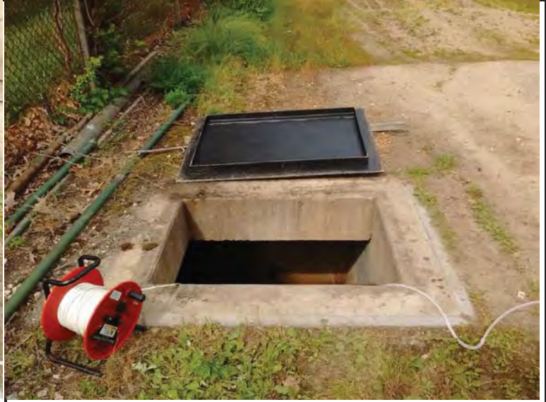
Photo 2. 3001-MW01 vault, showing surface runoff potential.
