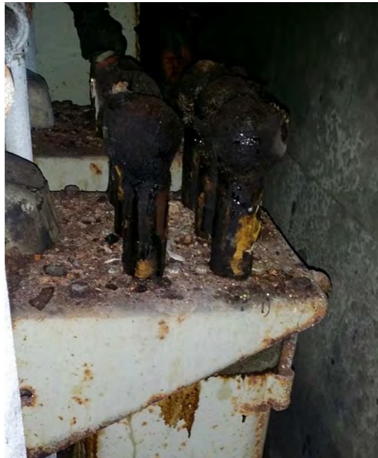
Battery 113. Partial cable components of the former transformer in the Electric Room of Battery 113, June 2016.
