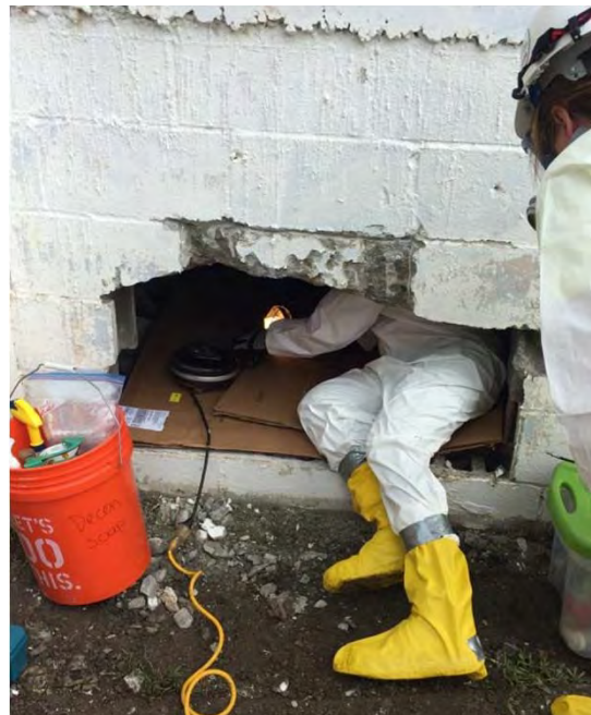
Battery 113. Hazardous materials survey team entering Battery 113 with lights, sampling equipment, and other supplies, June 2016.
