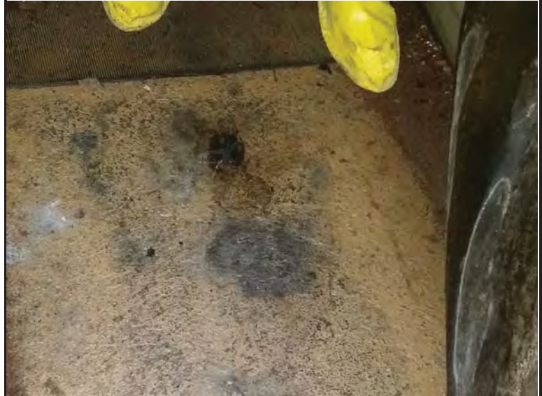
Photo 10. Floor staining in Transformer Room (Battery 113). One concrete chip sample was collected here (B113-CC01-01) for analysis of PCBs.
