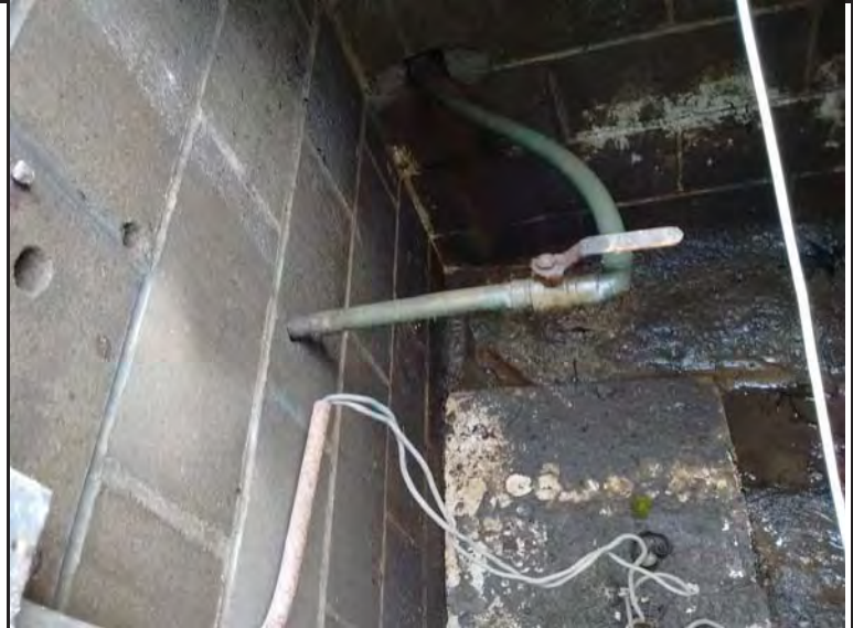
Photo 4. 3001-MW01, municipal water supply line and prior holes for well supply line.
