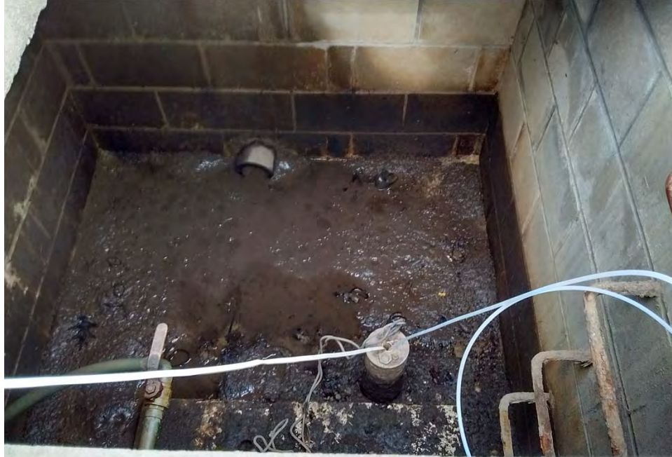
Existing well at Building 3001. Inside of the vault for the existing well at Building 3001, showing 4-inch casing with a 1-inch PVC pipe, with 6-inch drain pipe, June 2016.
