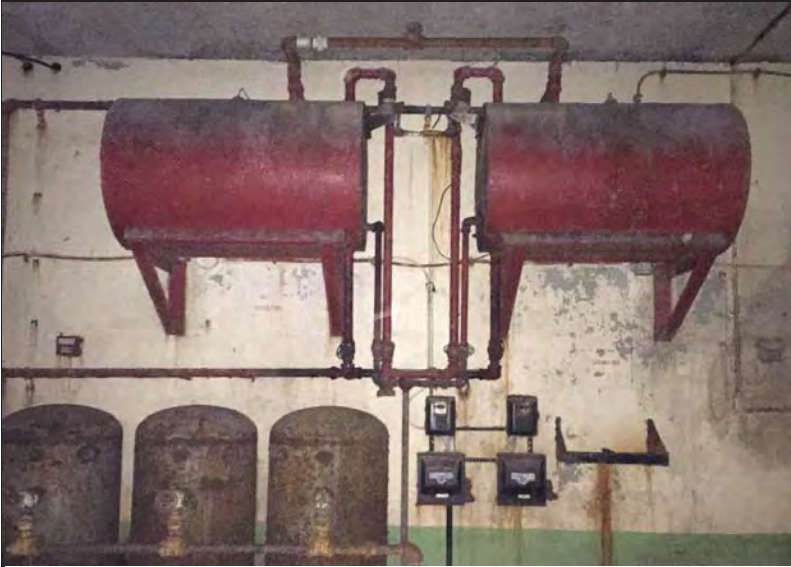
Photo 5. Storage tanks with petroleum product inside Battery 113. One liquid characterization sample was collected here (B113-LC01-01). The contents are suspected to be weathered diesel or fuel oil.
