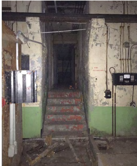
Battery 113. Stairwell and hallway from main hallway in Battery 113 to the Power Room, with rotten wooden floorboards near foot of stairwell, June 2016.
