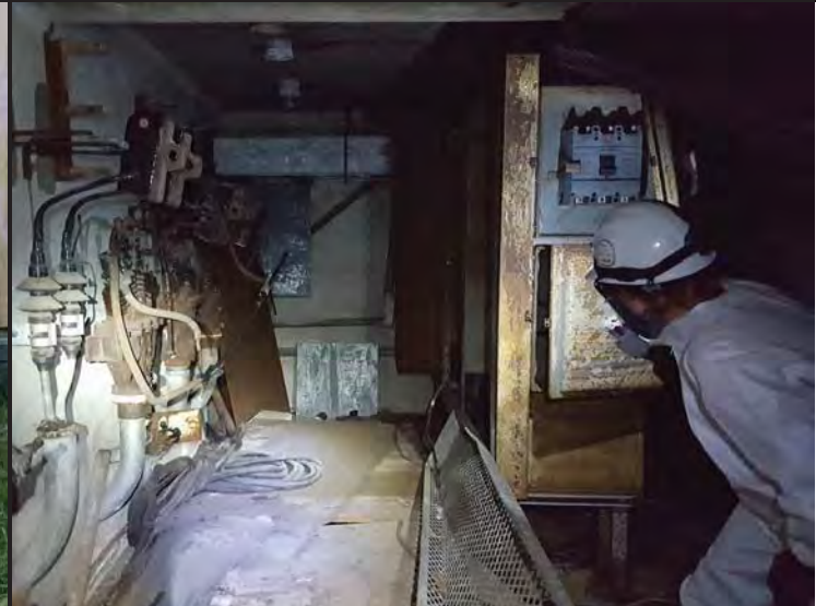
Photo 4. "Transformer" on wall in basement of Building 107 (Electrical Substation). Please also see photo 5 below, after inspection of the units, these features on the wall may be more appropriately labeled as electrical distribution boxes. Transformers were formerly located outside the building on nearby pads which were previously properly decommissioned.
