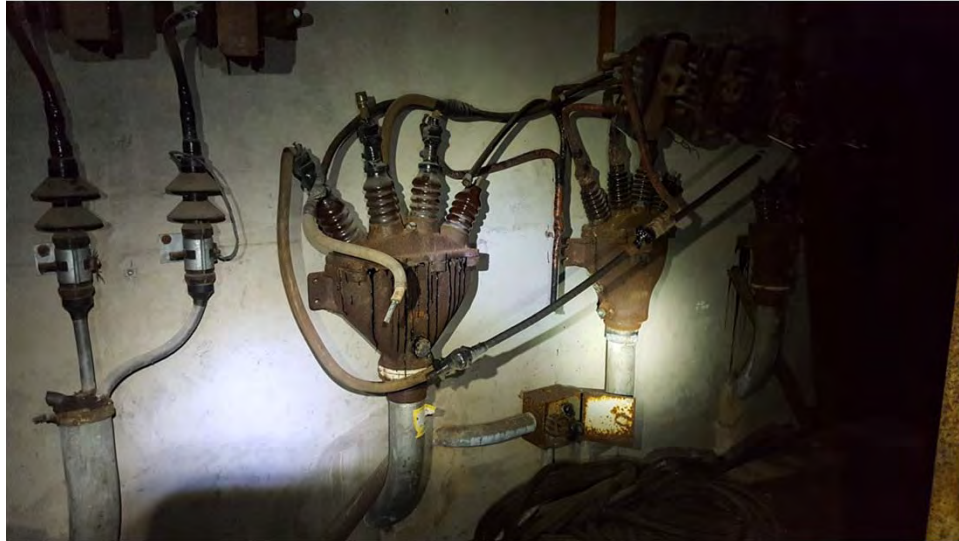
Building 107 (Electrical Substation). Portions of the former transformer, including a medium voltage cable breakout, June 2016.
