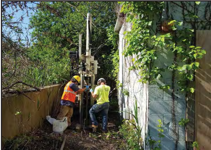
Photo 3. New England Geotech collecting soil core at AST35 with Direct Push Geoprobe 6620.
