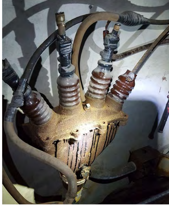
Building 107 (Electrical Substation). Close-up of a medium voltage cable breakout with dried oil, June 2016. One wipe sample was collected from the surface.
