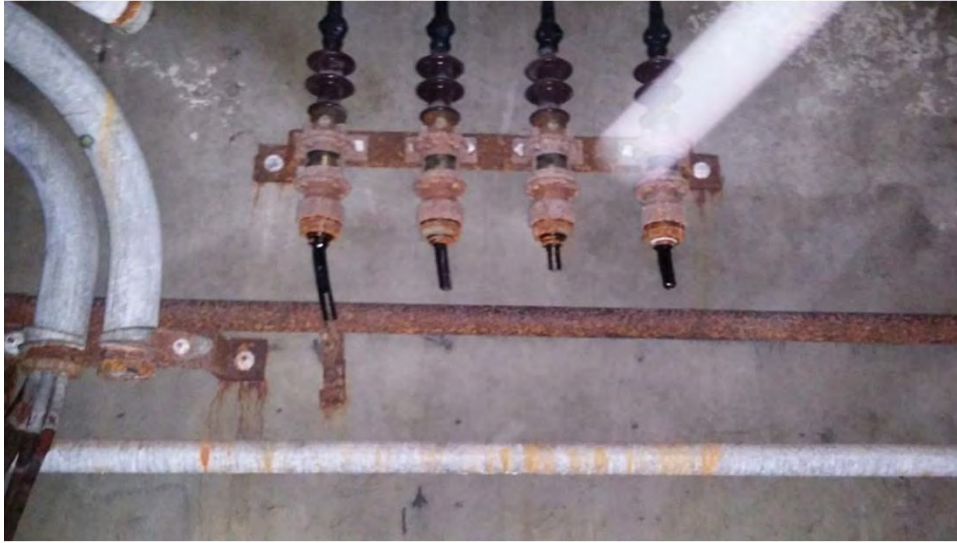
Battery 113. Partial cable components of the former transformer in the Electric Room of Battery 113, June 2016.
