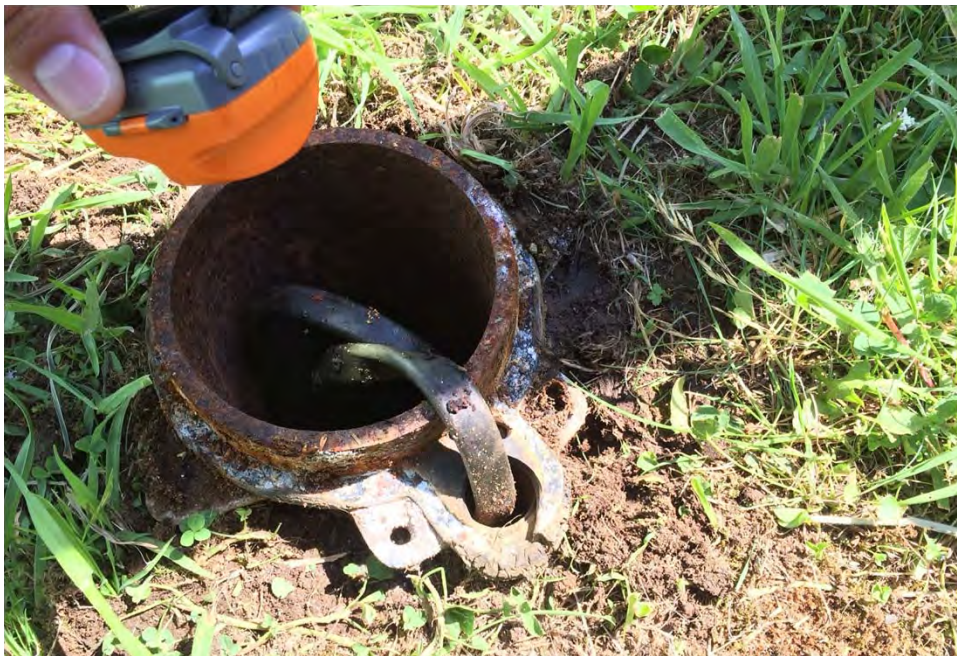
Motor Pool. Existing well at the Motor Pool near active ASTs, June 2016.
