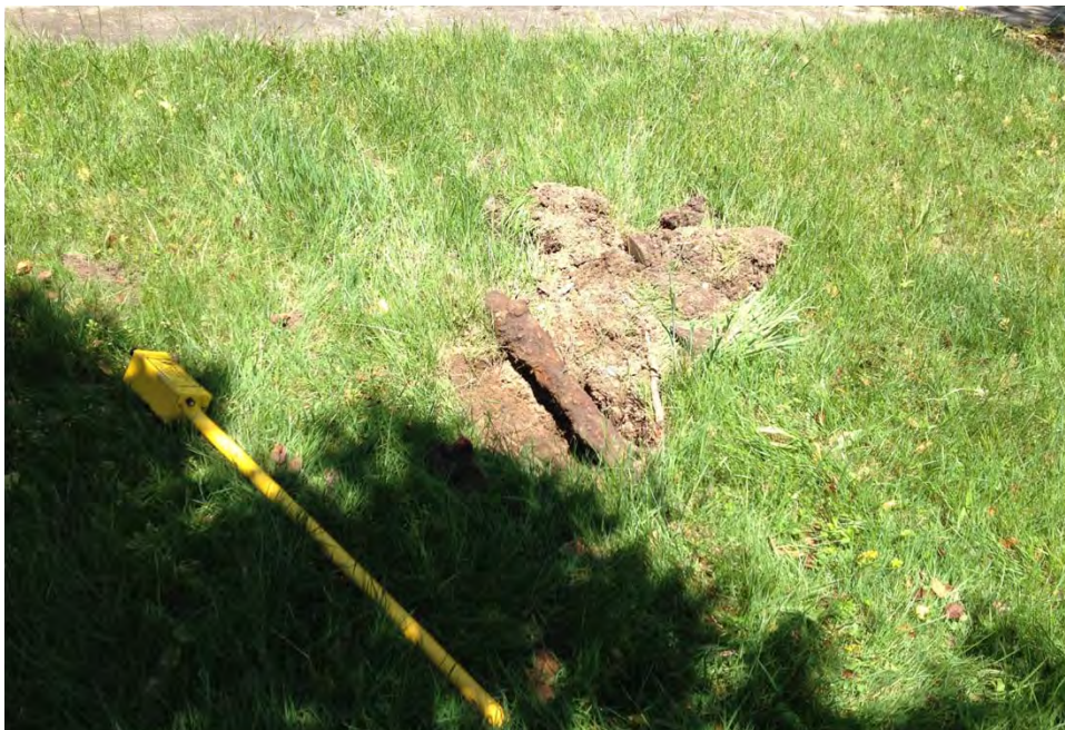
Suspected Tank C (former Building 2). Pipe uncovered while conducting "test holes" at the suspected tank C location, June 2016.
