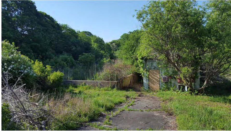
Fuel Pump House/AST 35. View of the former AST 35 containment area and the Fuel Pump house from the North, with sample locations flagged, June 2016.
