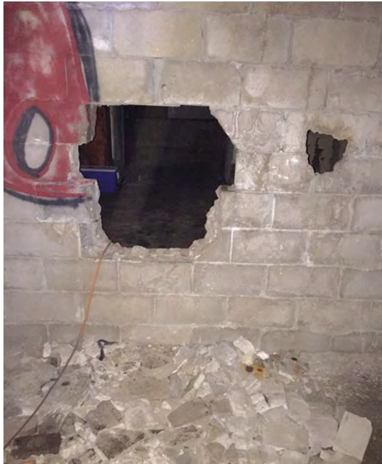
Battery 113. Access to main hallway of Battery 113 from entryway, June 2016. This demolition was already present when the team entered the Battery.
