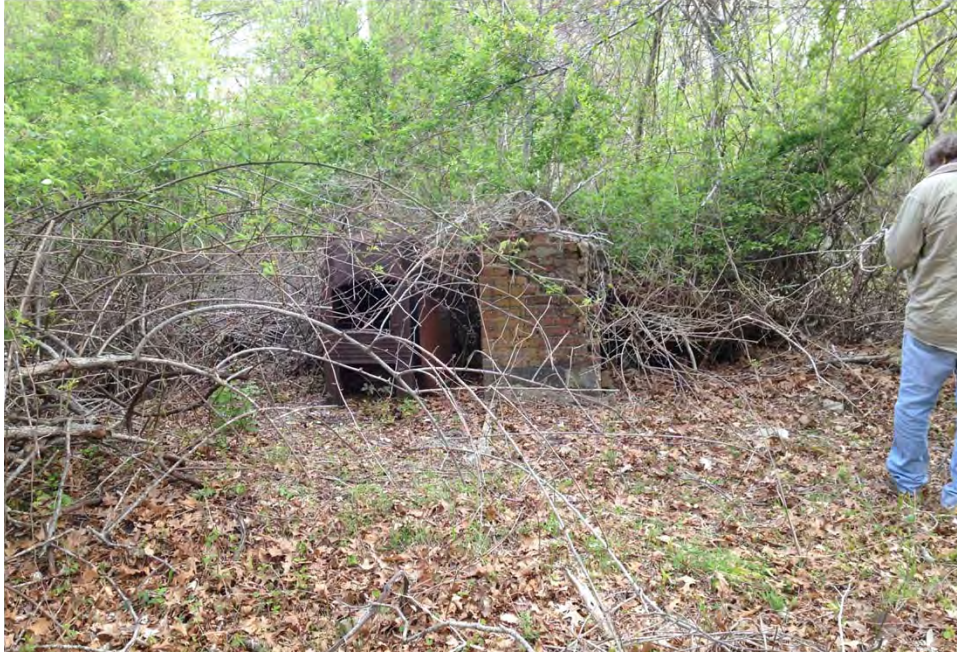
Former Building 034. Debris at former Building 034, which led to development of an additional AOC, May 2016.
