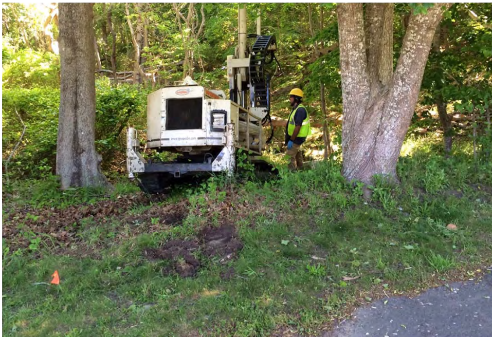
Waste Disposal System. Advancing boring WDS-SB07, June 2016. Location was relocated across the street due to identification of a suspected septic tank.
