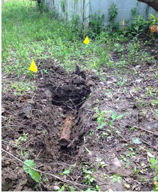
Fuel Pump House/AST 35. The end of the former fuel distribution line at the Fuel Pump House, identified by Shondstadt® magnetometer, June 2016.
