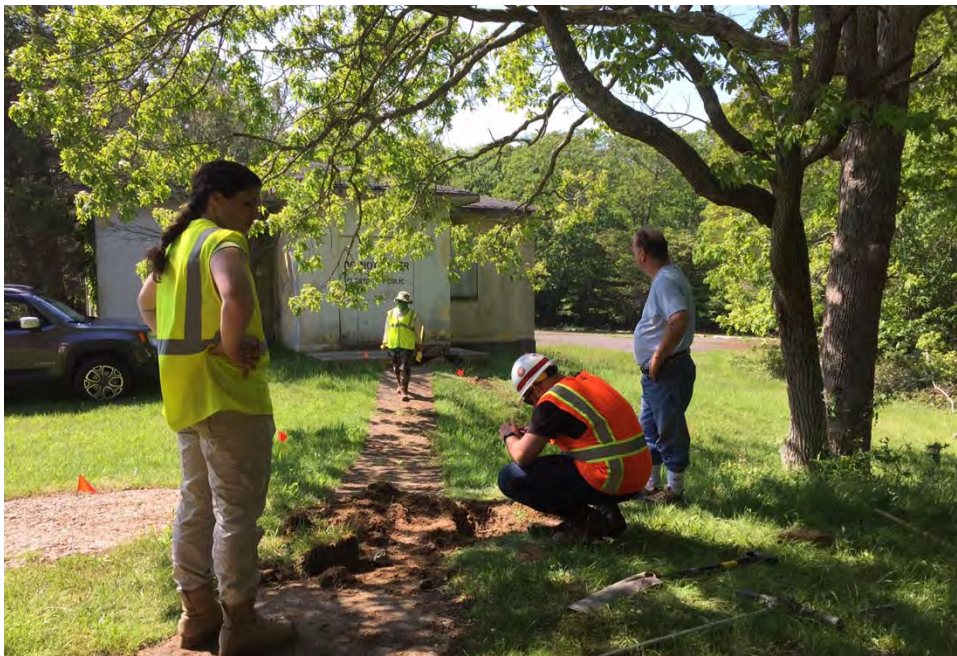
Suspected Tank H (Building 109). "Test holes" were conducted in June 2016, to investigate anomalies identified in the May 2016 geophysical survey.
