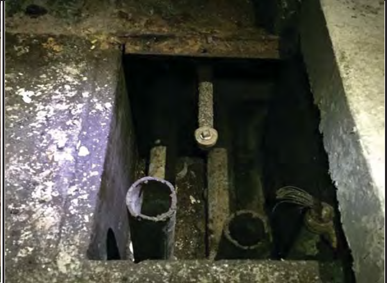
Photo 6. Piping under wooden floorboard in tank room of Battery 113. No tanks were identified in the trenches.
