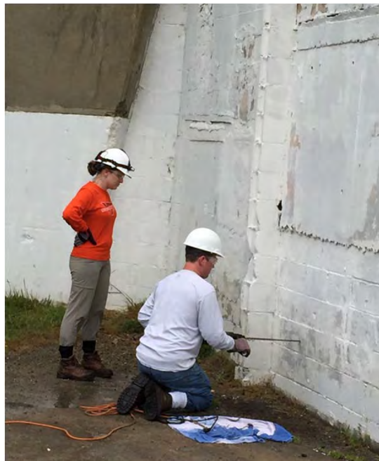
Battery 113. Chris Gamble (CGE) begins demolition of the entrance to Battery 113 with a demolition drill, June 2016.
