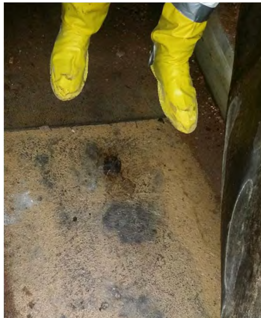
Battery 113. Floor staining in Electric Room of Battery 113 which was the location of concrete chip sample B113-CC01-01, June 2016.
