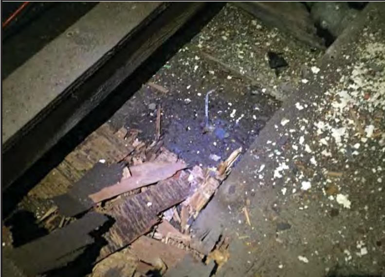
Photo 7. Rotting wooden floorboards over piping inside tank room (Battery 113).
