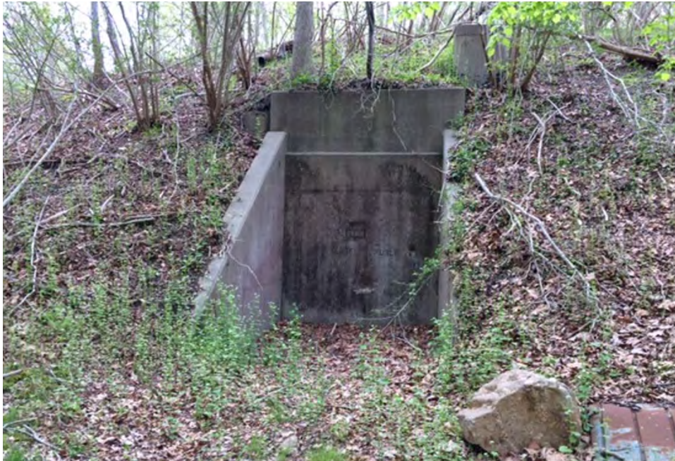
Plotting Room 113. Entrance to Plotting Room 113. Metal debris was located nearby via magnetometer survey in May 2016; sampling was conducted in June 2016.
