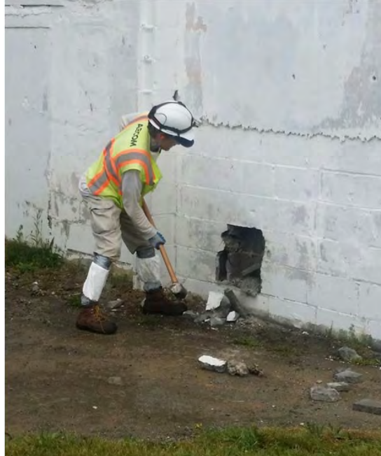
Battery 113. John Schroeder (AECOM) progresses demolition of the entrance to Battery 113 with a sledge hammer, June 2016.
