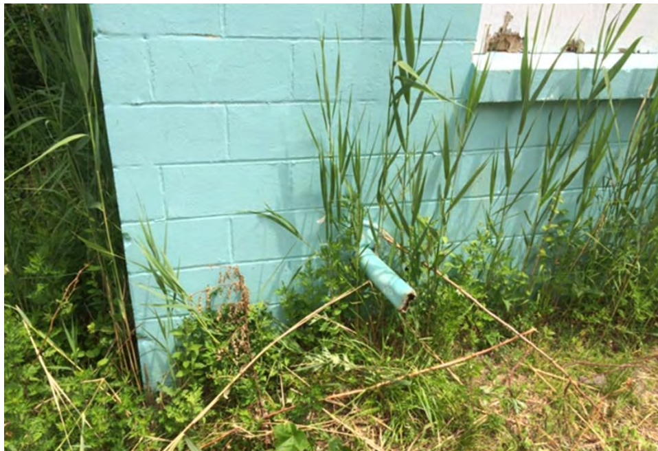
Building F100C. Piping at Building F100C, June 2016.
