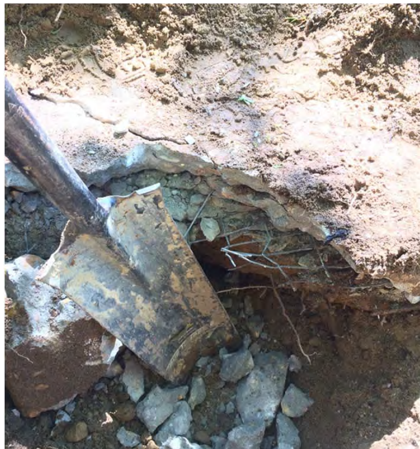
Suspected Tank H (Building 109). Wire mesh and rebar identified in "test holes" to investigate anomalies identified in the May 2016 geophysical survey, June 2016.
