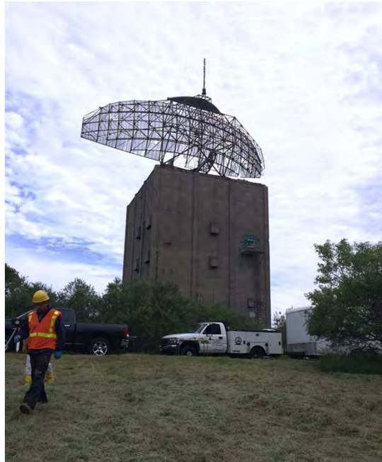
Building 203. Drilling equipment parked at former Building 203 beside the Radar Tower (Building 201), June 2016.
