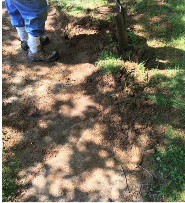
Suspected Tank H (Building 109). Backfilled "test holes" at suspected tank H, June 2016.
