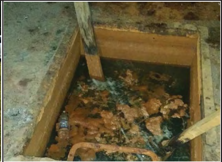
Photo 4. Standing water in pit near entrance inside Battery 113. (This pit was not sampled).
