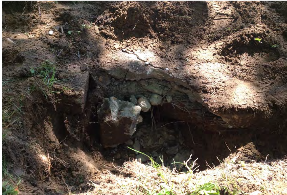
Suspected Tank H (Building 109). Wire mesh and rebar identified in "test holes" to investigate anomalies identified in the May 2016 geophysical survey, June 2016.
