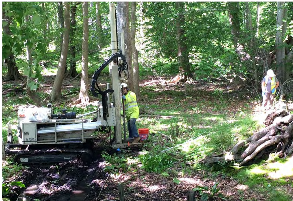
Waste Disposal System. Soil core collection from a waste disposal system location via the Direct Push 6620DT rig by Keith Precious (NEG), June 2016.
