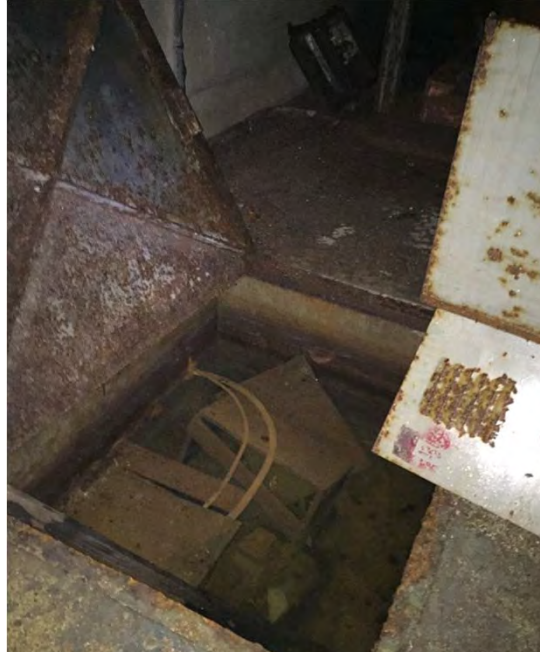
Battery 113. Pit with standing water in Battery 113. Liquid characterization sample B113-LC02-01 collected at this location, June 2016.
