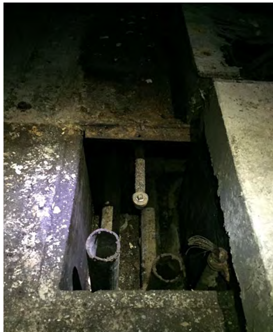
Battery 113. Trenches with piping in the Power Room of Battery 113, June 2016.
