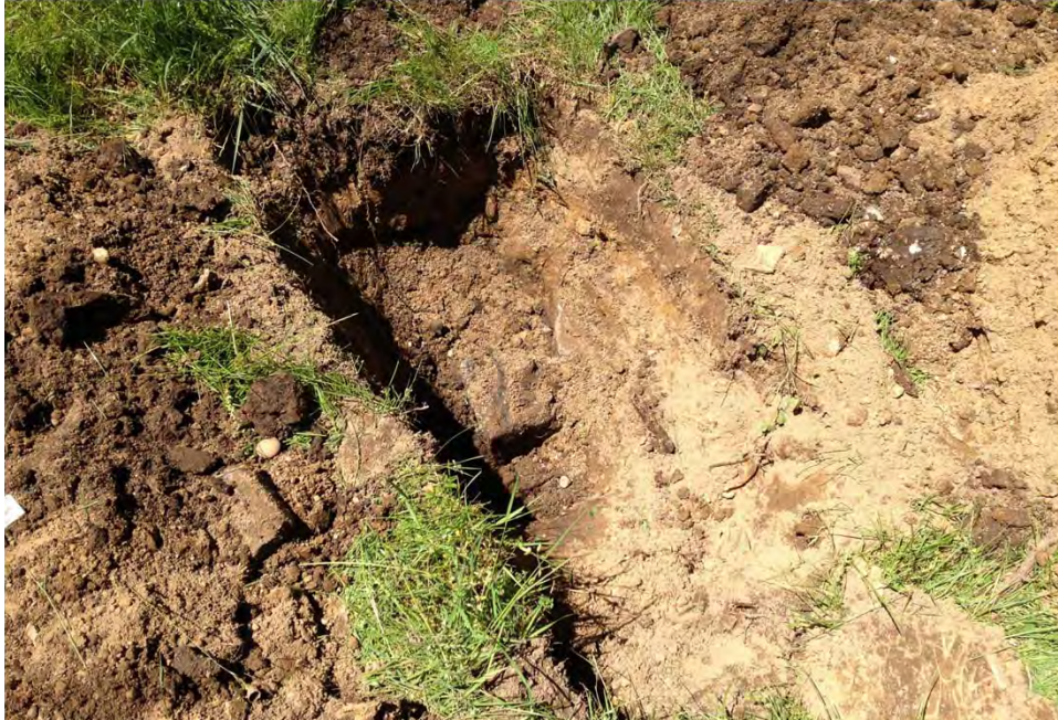
Suspected Tank C (former Building 2). Building debris uncovered while conducting "test holes" at the suspected tank C location, June 2016.
