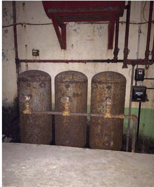
Battery 113. Three extremely rusted, unlabeled cylinders present below ASTs 3 and 4; the cylinders appeared to be empty, June 2016.
