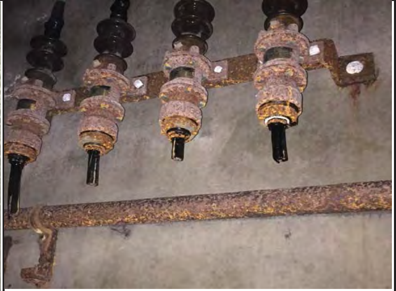
Photo 8. Portion of conduits with oil dripping in Transformer Room (Battery 113). One wipe sample (B113-WP01-01) was collected here for analysis of PCBs.
