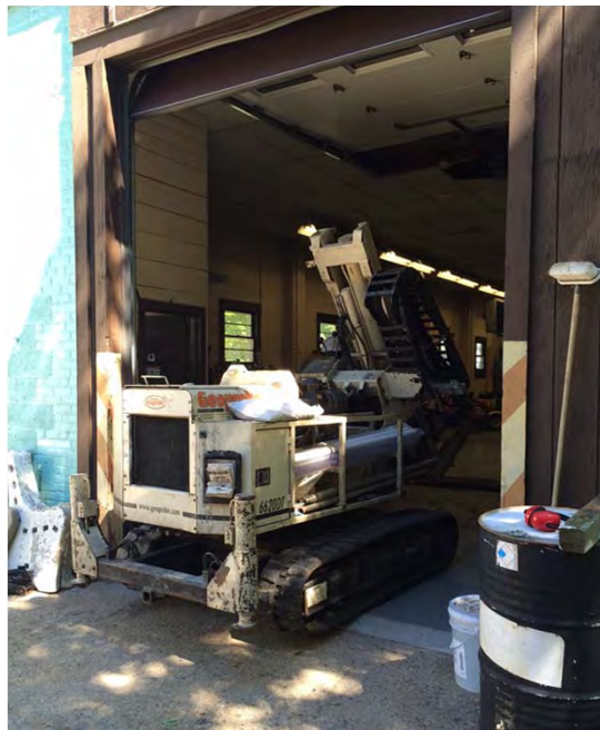
Motor Pool. Soil core collection from location MP-SB01 inside the Motor via the Direct Push 6620DT rig by NEG, June 2016.
