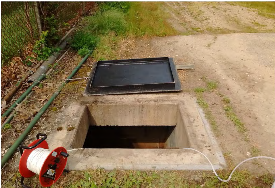
Existing well at Building 3001. Vault for historic water well at Building 3001, showing surface runoff potential, June 2016.
