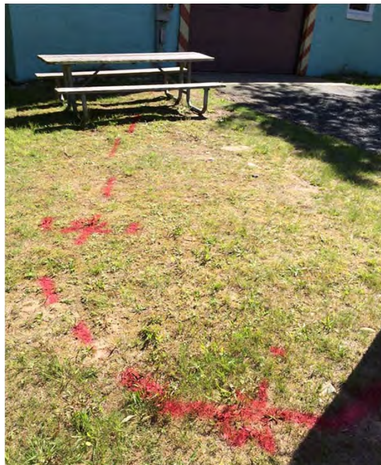
Motor Pool. Marked electric lines from the utility clearance at the Motor Pool, June 2016.
