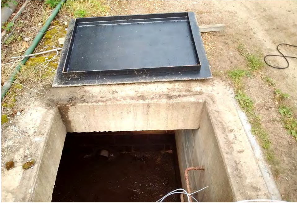
Existing well at Building 3001. Vault for historic water well at Building 3001, showing the confined nature of the space, June 2016.
