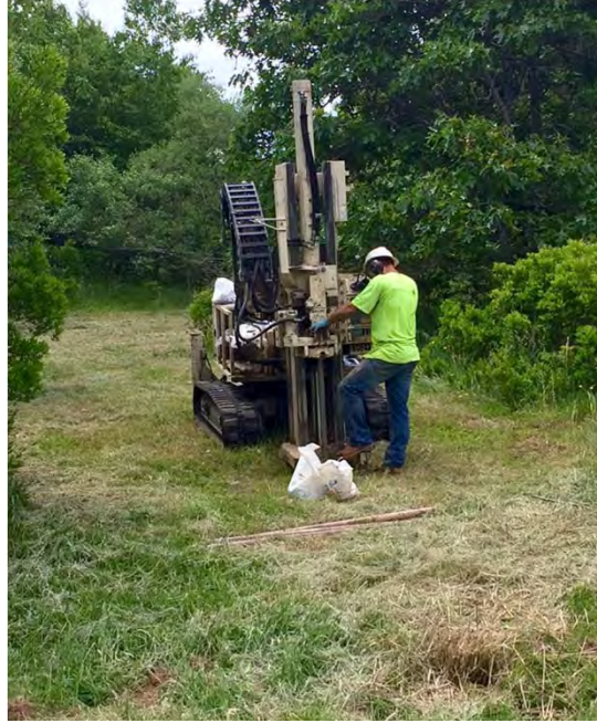
Former Building 203. Soil core collection from location 203-SB02 with the Direct Push 6620 DT rig by New England Geotech (NEG), June 2016.
