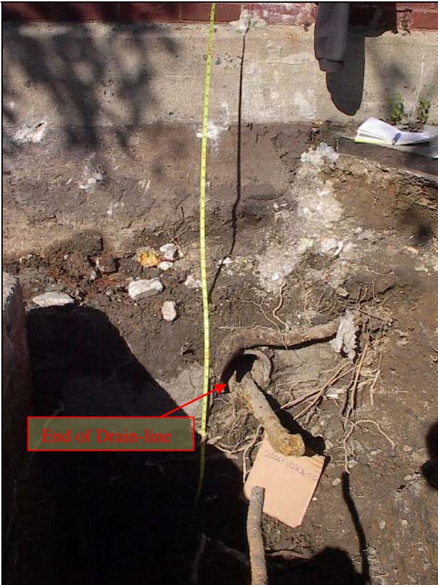
Photo 1 - Probable End of Drain-line
