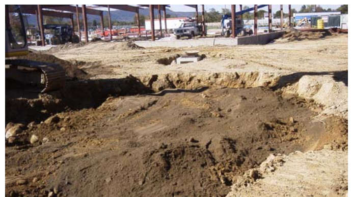
Project coordination and cooperation allowed the cleanup of buried items and construction of the bus garage to occur at the same time.
