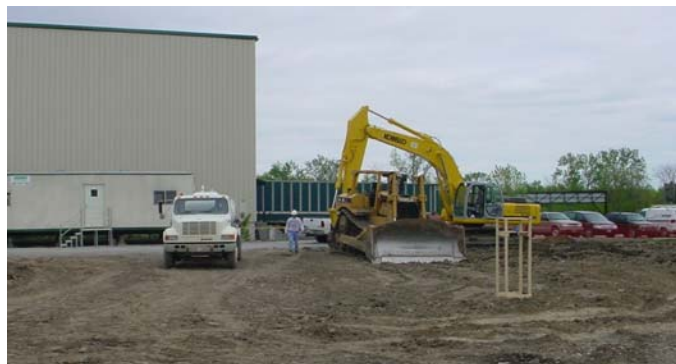
Heavy equipment was used to excavate over 2,800 tons of contaminated soil from the burn pit area cleanup.
