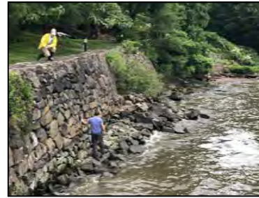
SEAWALL WASHOUT AND RIP-RAP
